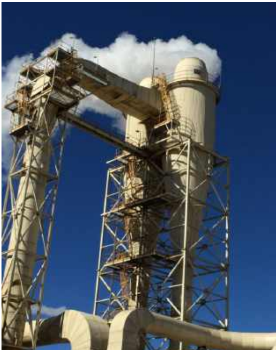
EPA 7 – Conti 2 Stage 1 Dryer Cyclone #1 (West) & EPA 8 – Conti 2 Stage 1 Dryer Cyclone #2 (East)
