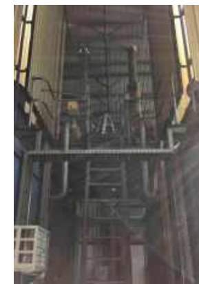
Cogeneration Plant 1 Stack & Cogeneration Plant 2 Stack
