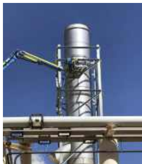
EPA 27 – Combined Conti 2 Press Vent Stack
