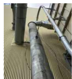
EPA 30 – Foam Station Baghouse
