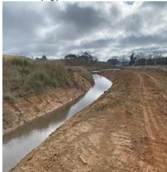
Swale conveying pond water to first flush basin
