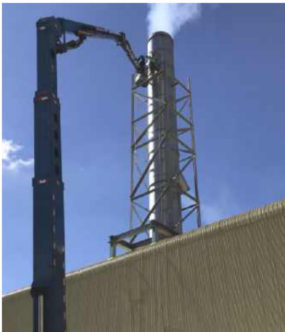
EPA 31 – Particle Board Press Extraction System
