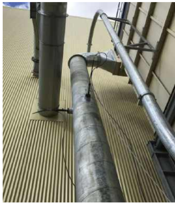
EPA 30 – Form Station Baghouse
