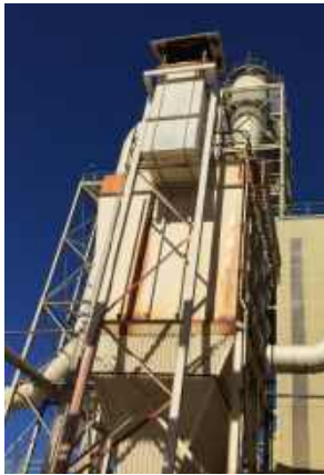
EPA 4 – DC1 Baghouse
