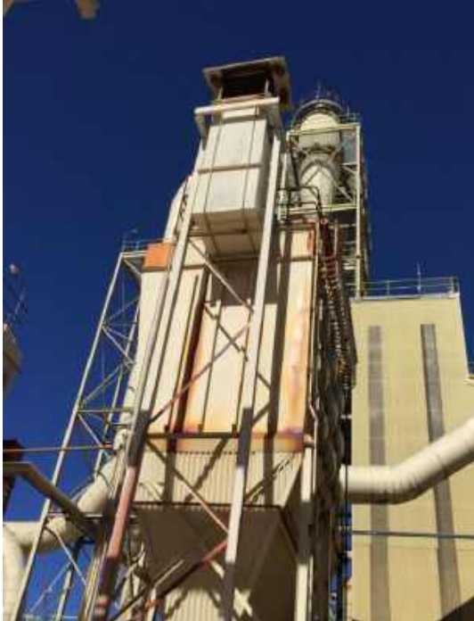
EPA 4 – DC1 Baghouse
