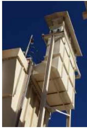
EPA 5 – DC2 Baghouse
