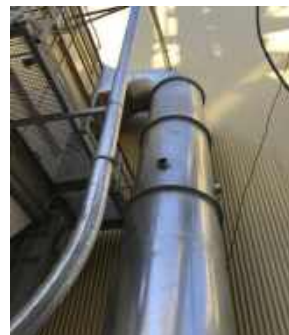
EPA 29 – Forming Line Baghouse
