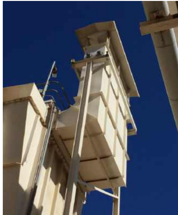
EPA 5 – DC2 Baghouse
